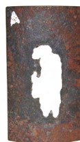
5" tubing 2 ⅝" PTC produced 2 holes 180° apart appx. flow area 3.75 in 2 (7.5 in 2 total)
